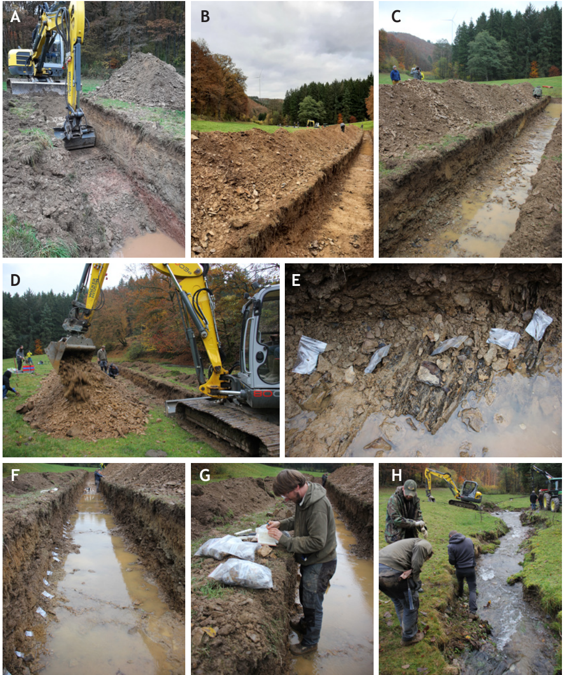
ANNEX II: A) Digging the fifth trench (V) on a higher part of the alluvial plain. Notice the colour shift in lithologies within the deposited alluvium. Unfortunately, no original strata were reached as a result of rising groundwater and vast deposits of unconsolidated alluvium. B) Main trench (I) freshly dug out. C) After a few moments groundwater was seeping into the main trench (I). D) Excavator separating the original bedrock from the alluvium. E) Sample bags along the freshly excavated original bedrocks within the primary trench (I). F) Sample bags along the side of the main trench sampling every 25 cm. G) Samples had to be recorded quickly and collected to prevent the rising groundwater from washing them away. H) Looking for the typical red fossiliferous concretions along the banks of the Fél stream.
